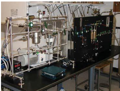
Gas Blending Manifold
