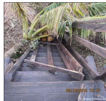
Cyclone Gita Damage at SMO February 2018
